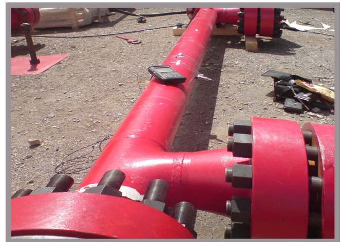
fig2. The natural gas pipeline in Spain.
