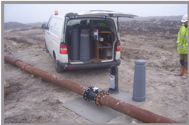
fig1. The ABB AquaMaster Installation.
