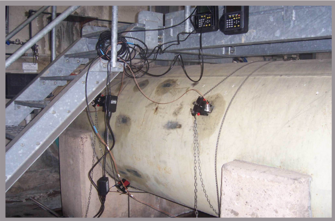
fig1. PT878 installed on the pipelines.
