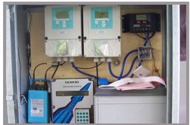
fig3. The equipment used. OCMIII and HydroRanger 200.
